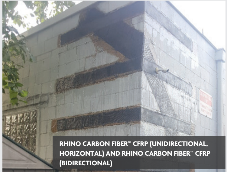
BLOCK WALL CORNER CRACKS FILLED WITH HYDRAULIC CEMENT
